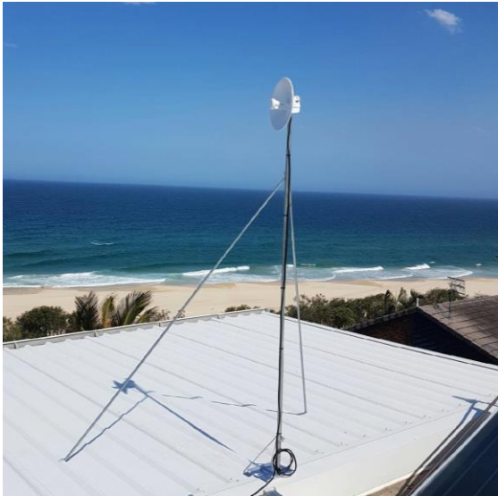
Installed pole with 300mm diameter dish
